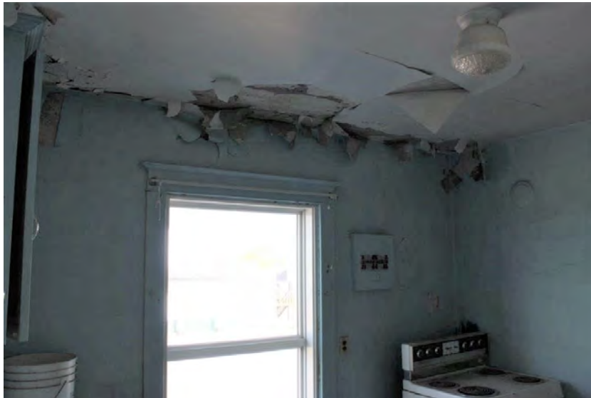
Photograph 12: Water damage on the second floor of the Seniors Center (June 23, 2021).
