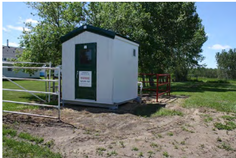
Photograph 6: The Paintearth Gas Co-op Ltd. metering station near the southwest portion of the Campground (June 23, 2021).
