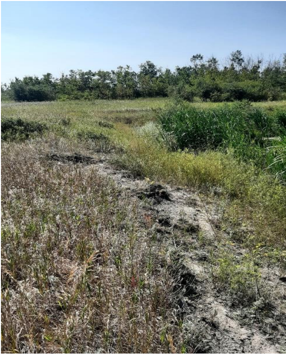
Figure 3.7: South Anaerobic Cell Erosion
