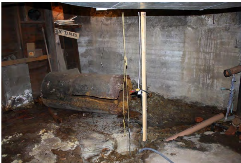
Photograph 6: A storage tank and sump in the Seniors Center basement, noting wet conditions, salt staining and deteriorating infrastructure (June 23, 2021).
