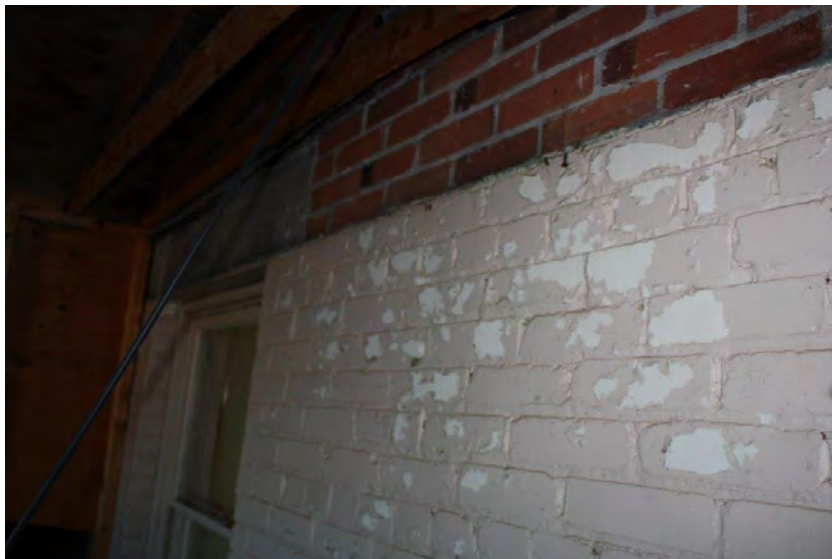
Photograph 14: Layered paint on a former external wall which has since been added on to with the addition of the Village Office (June 23, 2021).
