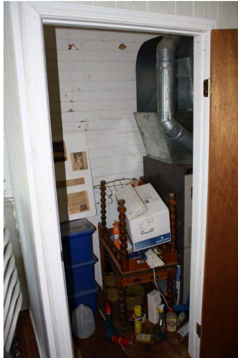
Photograph 3: The furnace in the mechanical room in the northwest portion of the Church (June 23, 2021).
