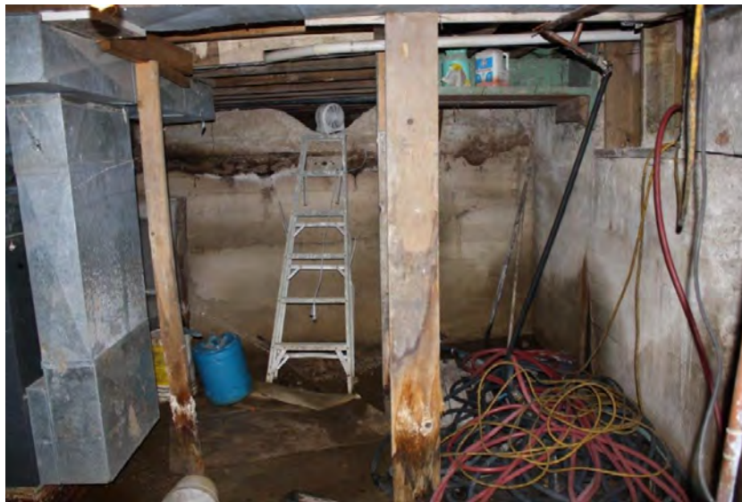
Photograph 8: The Curling Rink basement, noting the water wicking in the wooden pillar and poor condition of the infrastructure (June 23, 2021).
