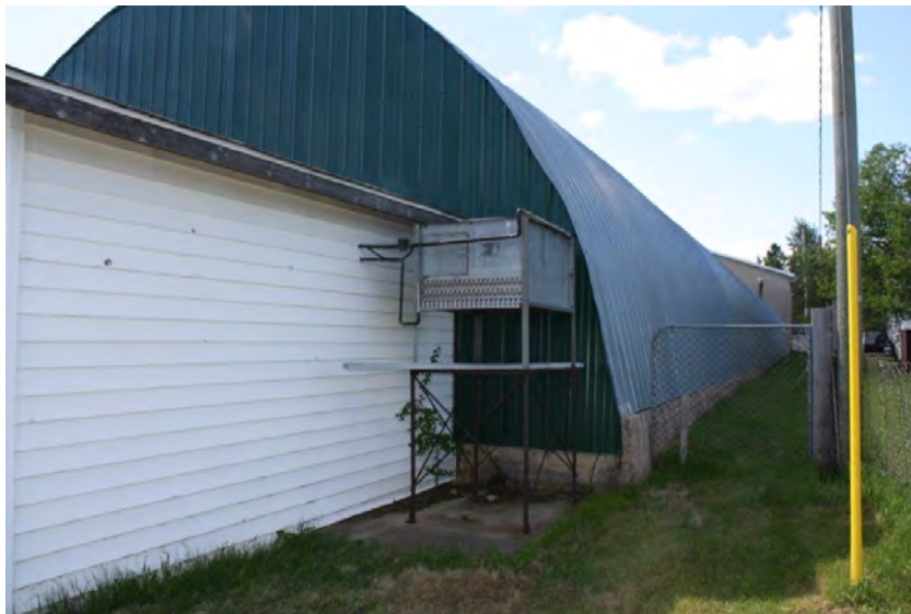
Photograph 12: Components of the artificial ice system, containing freon, west of the addition (June 23, 2021).
