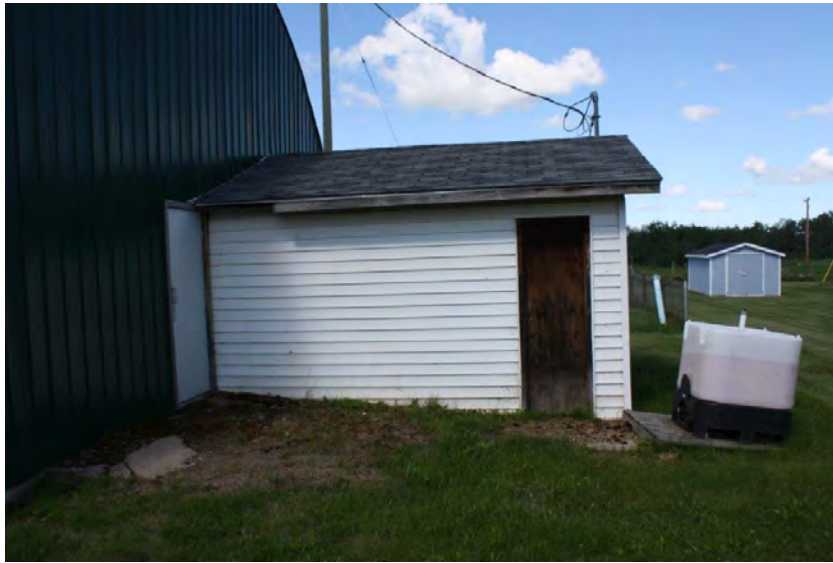
Photograph 11: The addition on the north side of the Curling Rink where the artificial ice system was located along with a plastic tote containing calcium chloride (June 23, 2021).
