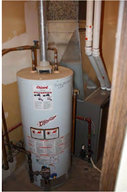
Photograph 19: The mechanical room in the Public Works shop which also services the Village Office (June 23, 2021).
