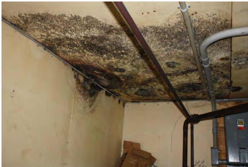
Photograph 14: Mould in the addition on the north side of the Curling Rink (June 23, 2021).
