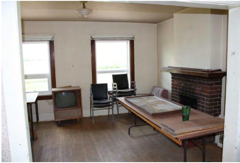
Photograph 11: The living room on the second floor of the Seniors Center (June 23, 2021).
