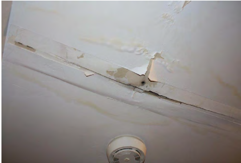
Photograph 31: Water damage in the ceiling of the Community Hall on the second floor (June 23, 2021).
