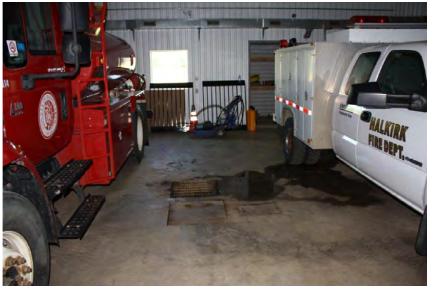
Photograph 40: The drain and sump in the original building at the Fire Hall (June 23, 2021).
