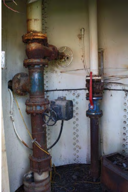
Photograph 35: Piping within the Water Tower (June 23, 2021).
