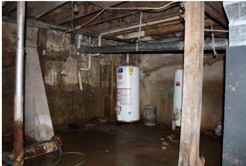
Photograph 7: The Curling Rink basement, noting the wet conditions (June 23, 2021).
