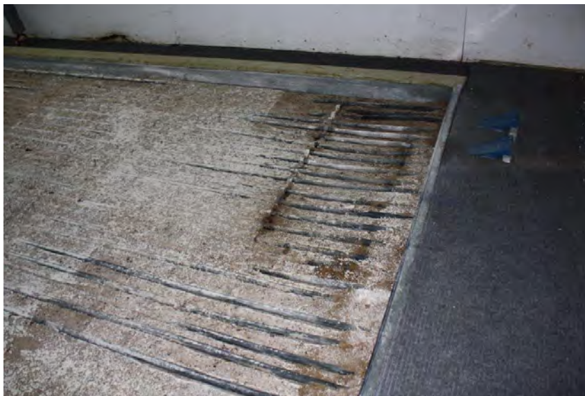
Photograph 10: A close up of the artificial ice system piping within the ice sheets (June 23, 2021).
