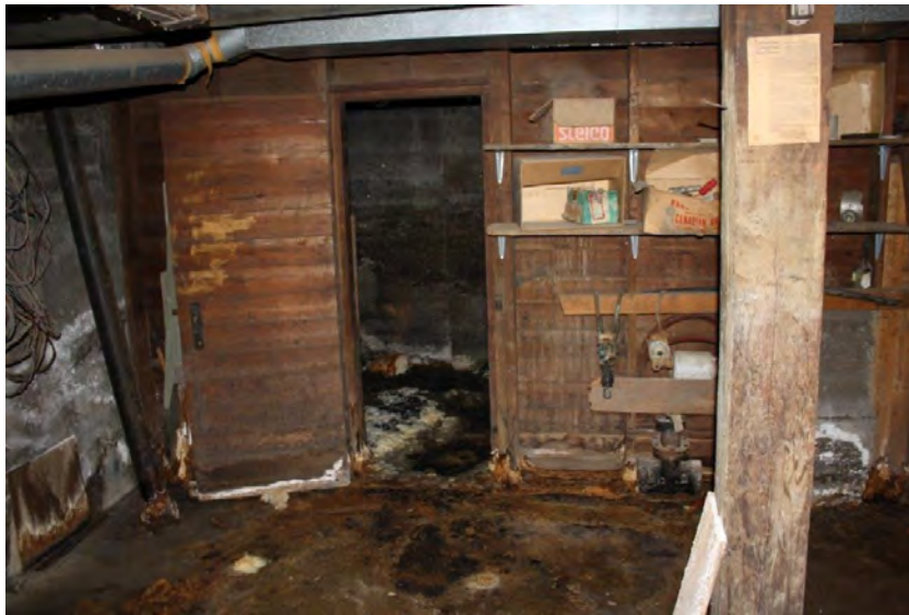
Photograph 5: The Seniors Center basement, noting poor conditions (June 23, 2021).
