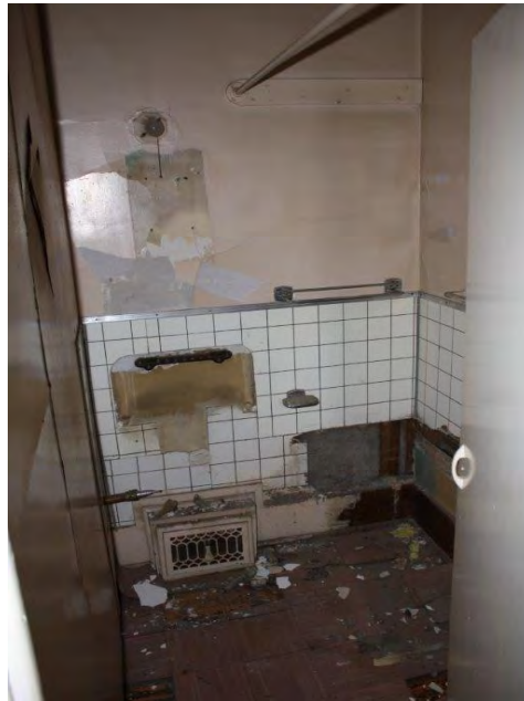
Photograph 13: The former washroom on the second floor of the Seniors Center (June 23, 2021).
