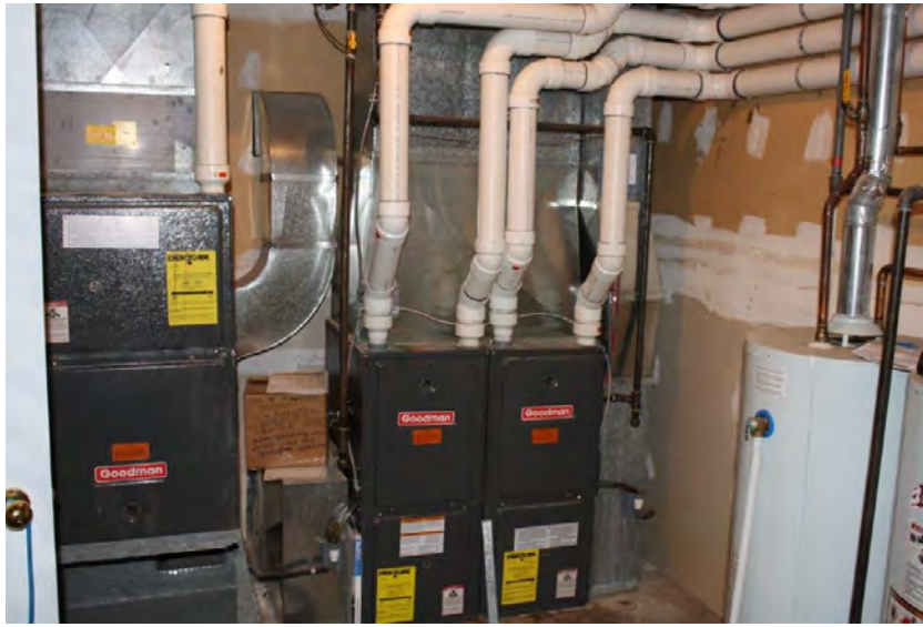
Photograph 29: The mechanical room in the basement of the Community Hall (June 23, 2021).
