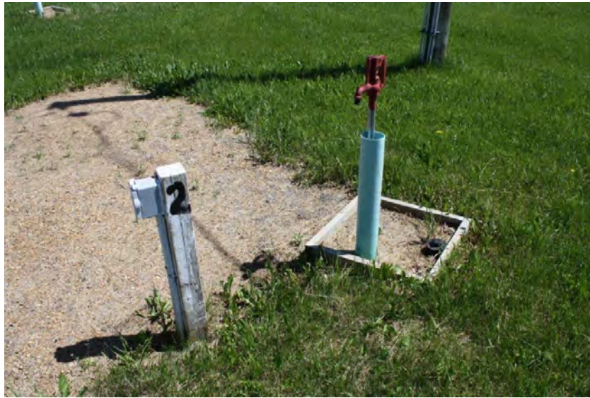
Photograph 3: Typical services including power, water and sewer at a stall within the Berry Street Campground (June 23, 2021).
