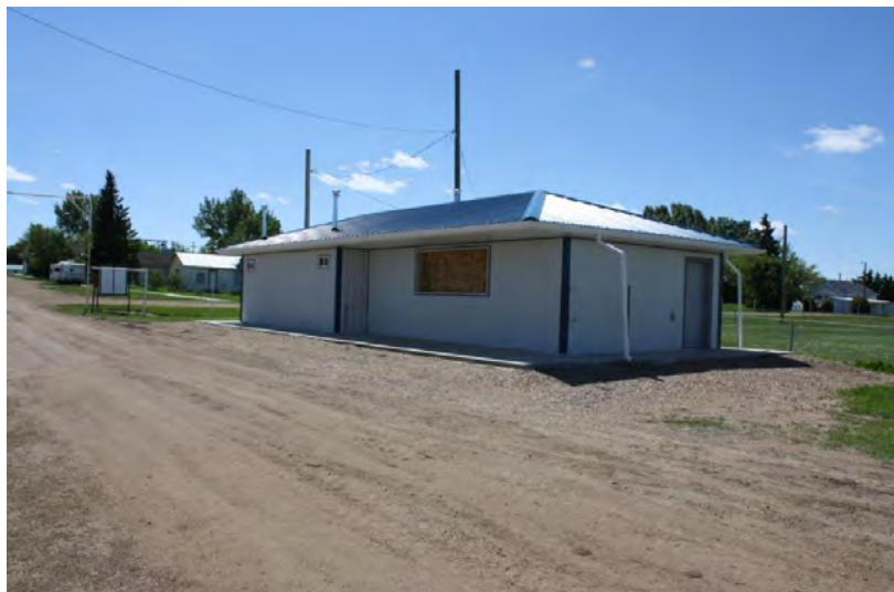
Photograph 4: Looking south at the new washroom and concession near the Main Street entrance of the Campground (June 23, 2021).
